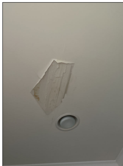
Damaged ceiling in hallway
