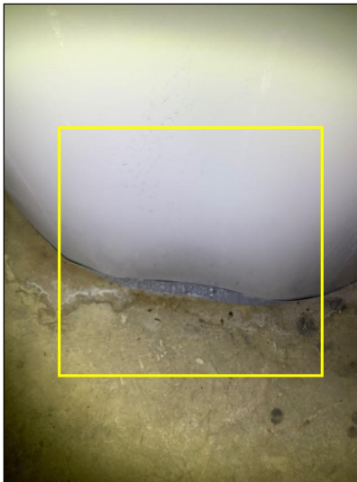
Dents observed throughout water heater enclosure
