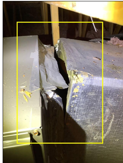
Return air vent detached at furnace in attic
