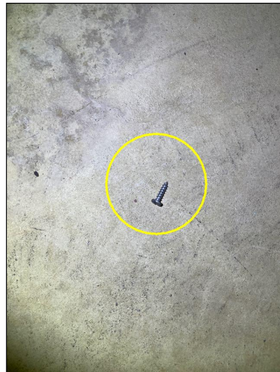
Sharp-pointed metal screws hold panel cover in place. These are a potential hazard as they may puncture wire insulation and electrify panel box, becoming a shock or electrocution hazard. These screws should be replaced with approved, flat-tipped screws.
