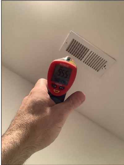
Supply air temp in heat mode 95 degrees
