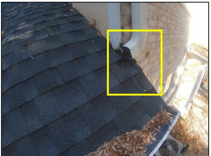
Downspout/s discharging on roof observed.
