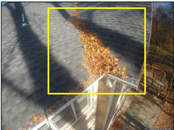
Clean roof areas: Significant amounts of organic debris evident.
