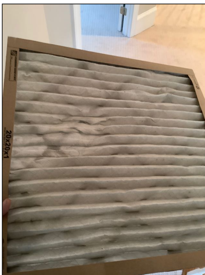
The filter is dirty. Needs replacement.
