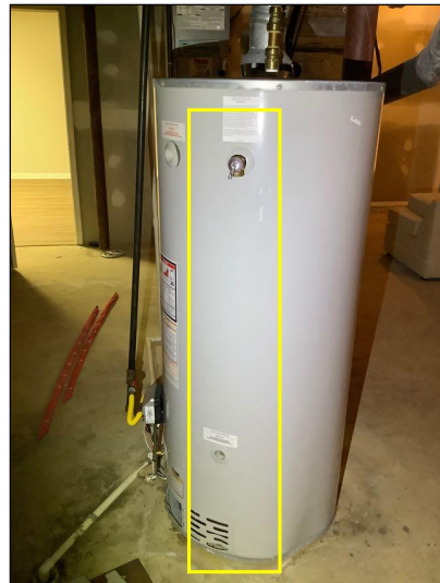
Extension missing from water heater TPRV
