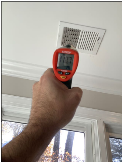
Supply air temp in heat mode 118 degrees
