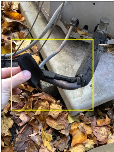
Deteriorated insulation on the refrigerant lines, replace as needed
