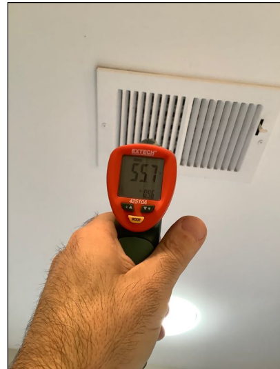
Supply air temp in cooling mode 55 degrees
