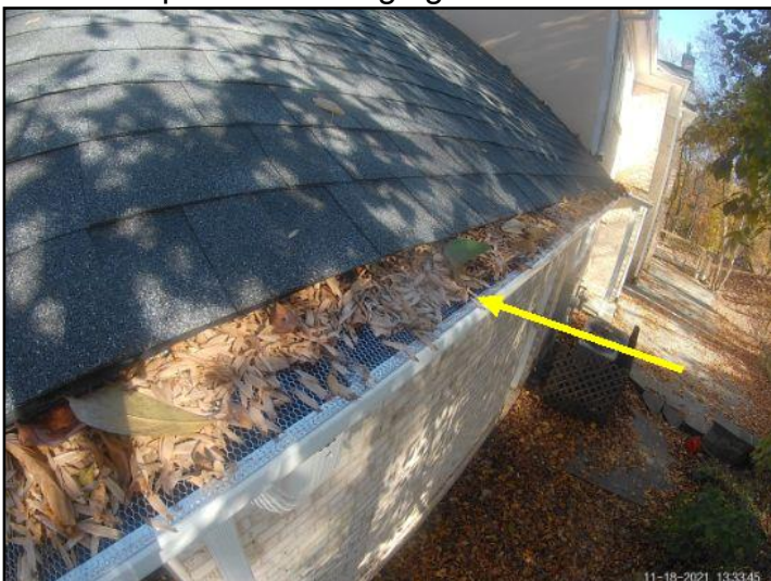
Debris noted in gutters. Recommend cleaning gutters so that water can properly drain.
