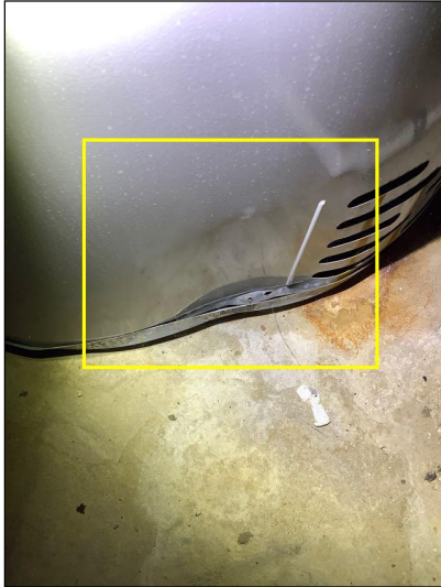
Dents observed throughout water heater enclosure
