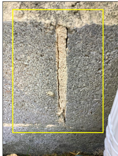
Cracks/deteriorated mortar observed. Recommend sealing/re-pointing as needed to prevent moisture intrusion.
