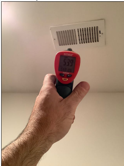
Supply air temp in cooling mode 53 degrees
