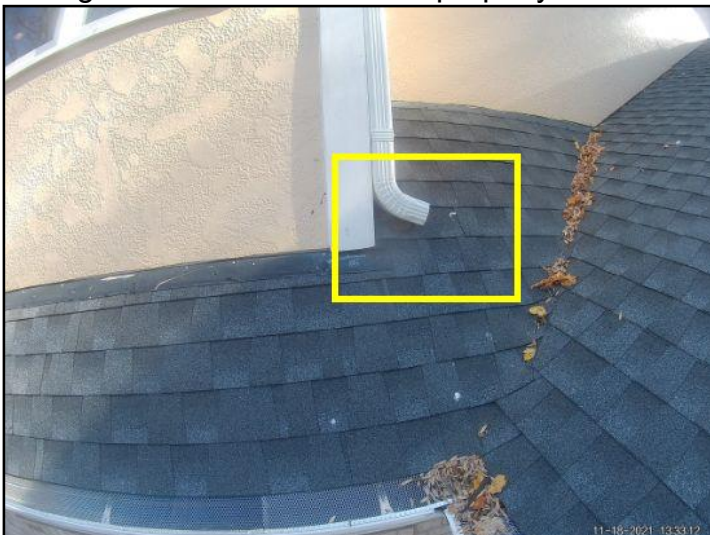
Downspout/s discharging on roof observed.
