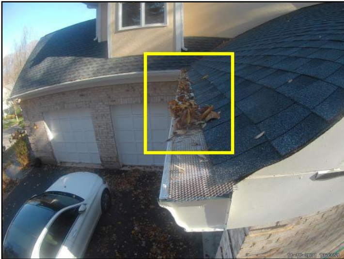
Debris noted in gutters. Recommend cleaning gutters so that water can properly drain.
