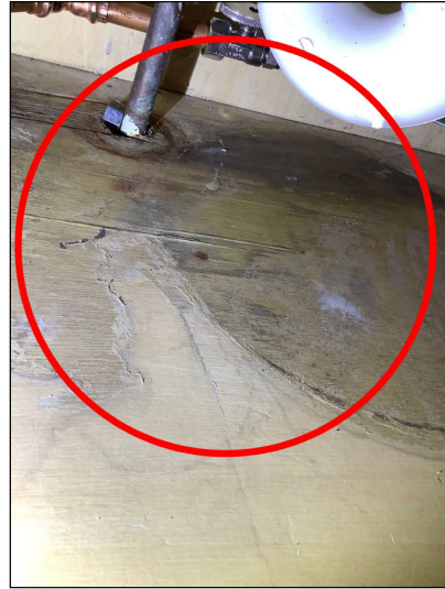
Evidence of previous/past leak noted, it is dry at the time of the inspection.
