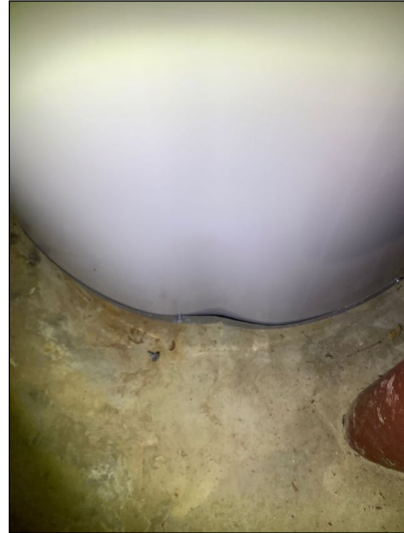
Dents observed throughout water heater enclosure
