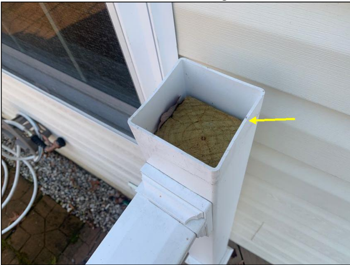
Post cover missing
