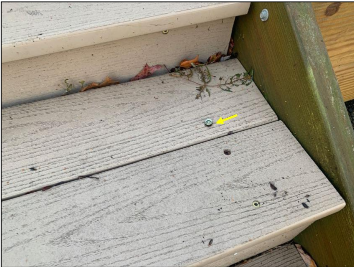
Loose nails and treads
