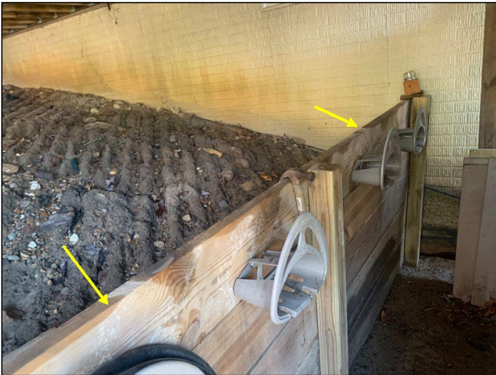
Retaining wall is loose; Posts are not secured to wall
