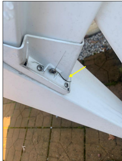
Cover piece missing over screws; Cracked railing
