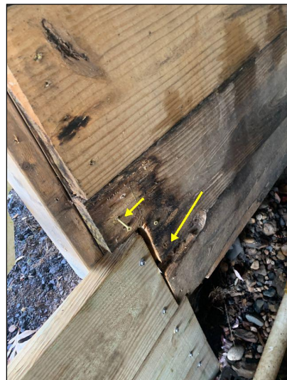
Loose screw; Deterioration wood at retaining wall under deck
