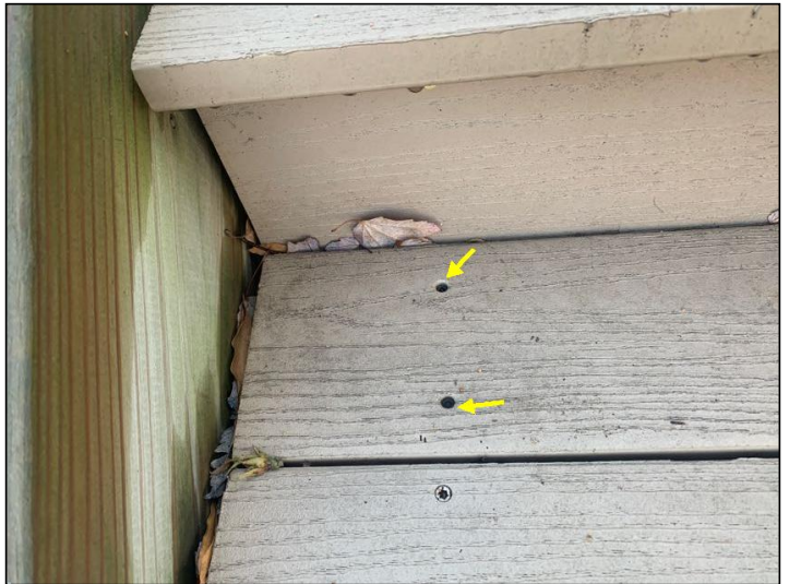
Nails driven in too deep
