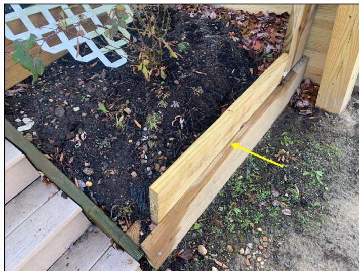
Loose retaining wall
