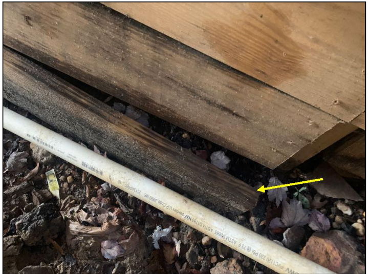
Retaining wall loose under deck
