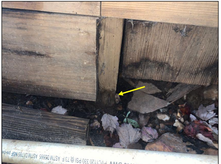
Post in contact with soil some deterioration noted
