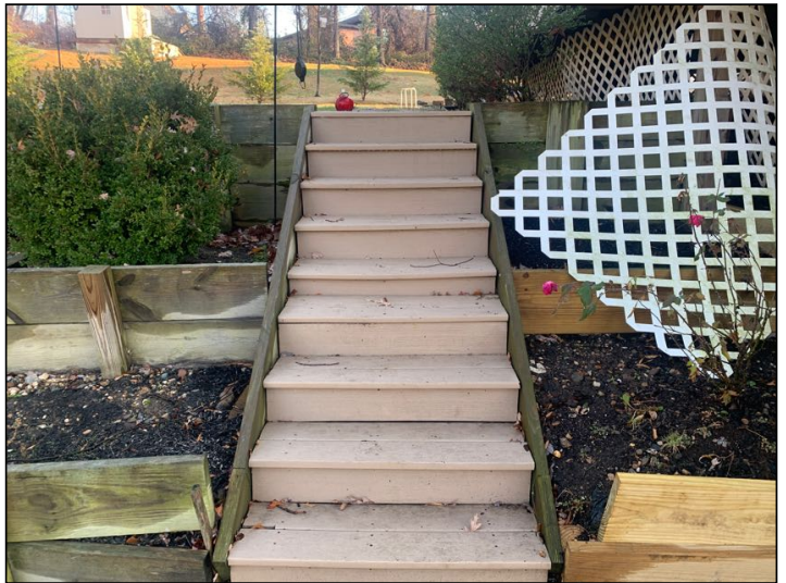
No railing; Risers vary greatly in height
