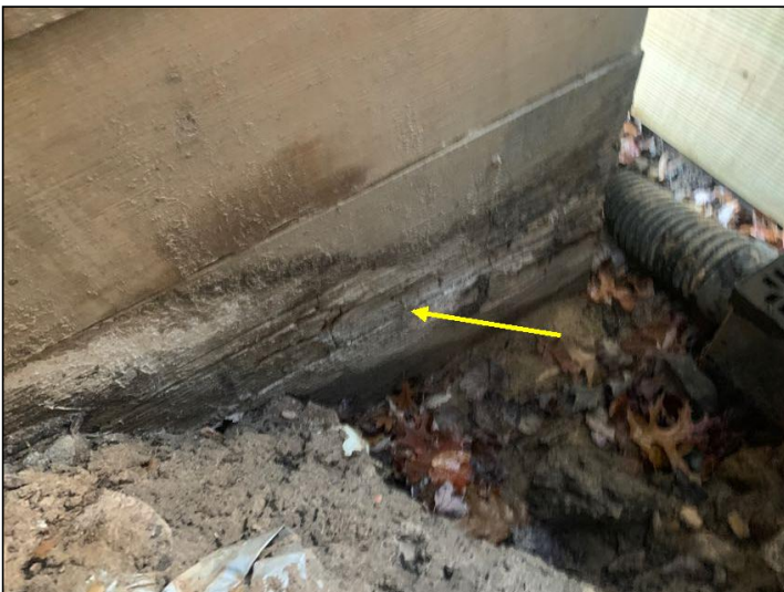
Deteriorated wood at retaining wall under deck
