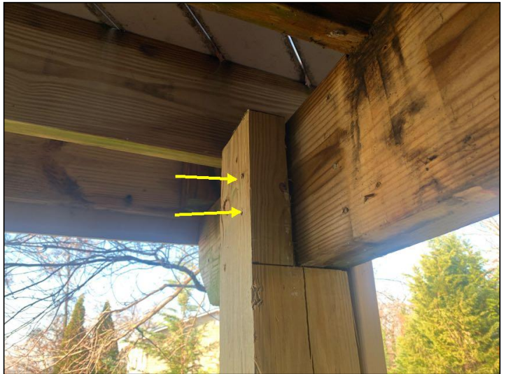
No lag bolts on any posts; Post not completely secure
