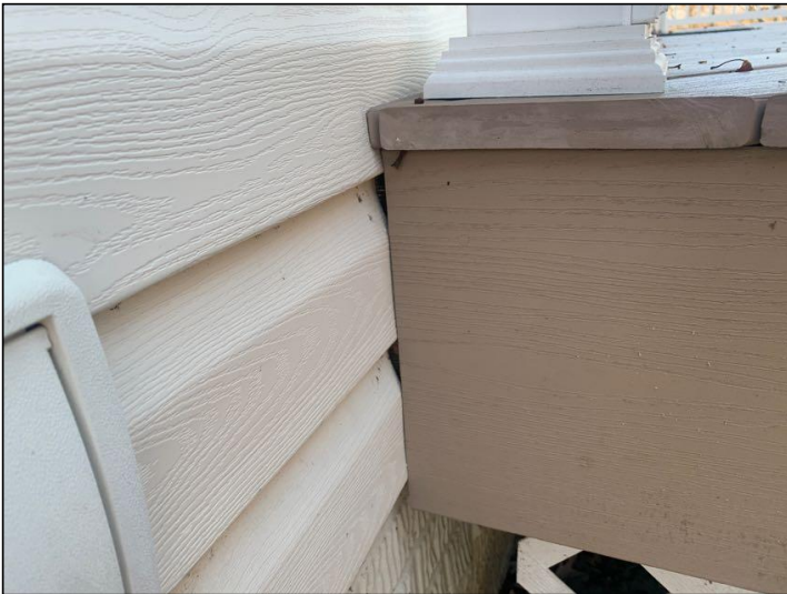
Deck not flashed; Installed directly over siding
