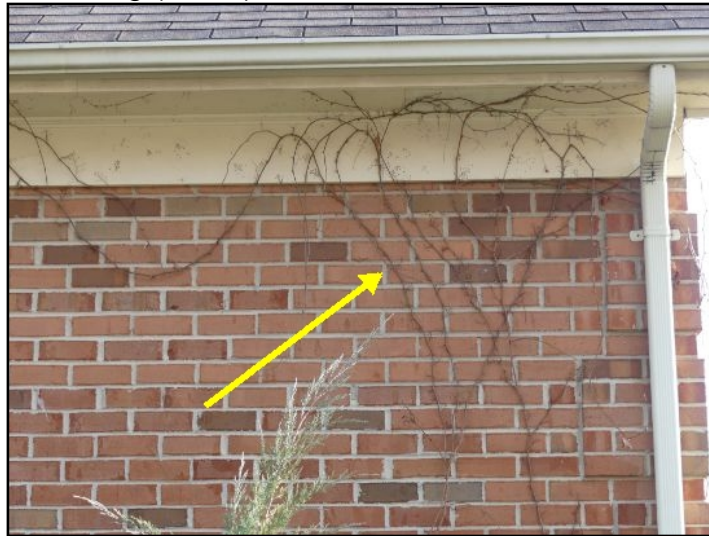
Vegetation on cladding
