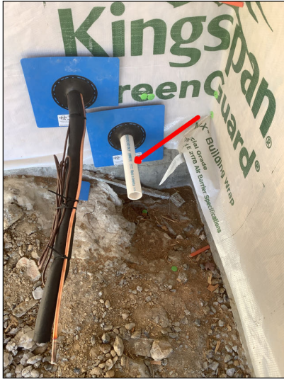
Sump pump discharge pipe
