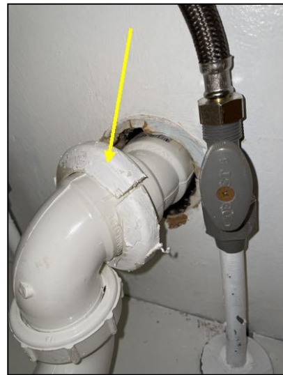
Loose and broken escutcheon
