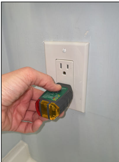
Now power to outlet
