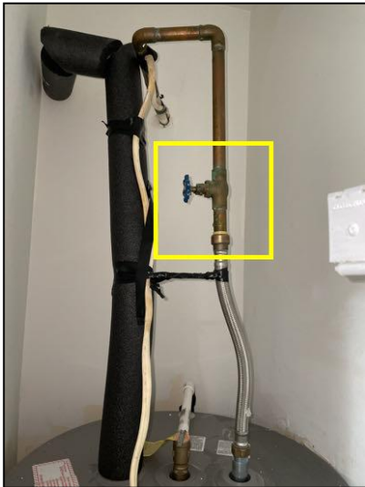
Water shut off valve
