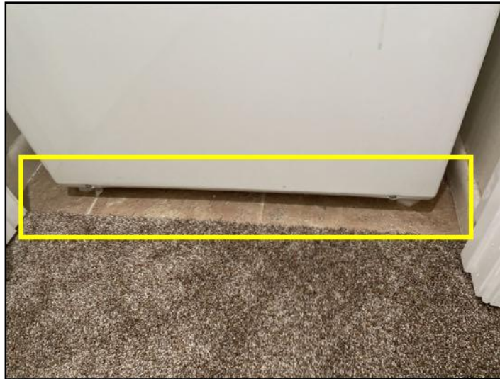
Missing overflow pan
