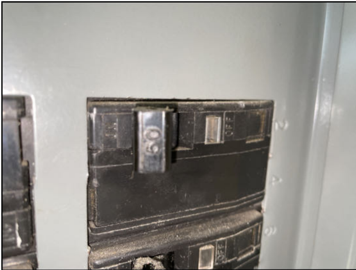
50 amp furnace breaker
