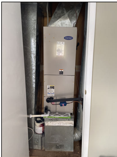
Missing shut off switch
