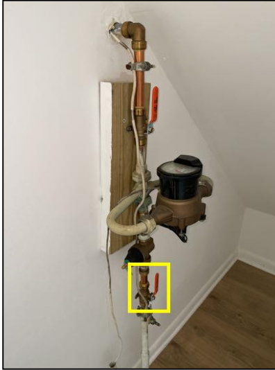
Main water shut off valve
