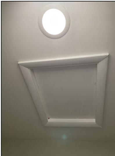
Plumbing access panel
