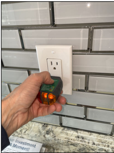
Not GFCI protected
