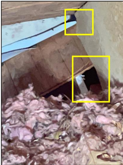
Gaps in firewall
