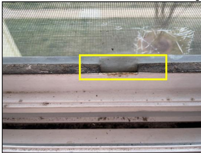
Deteriorated glazing bead
