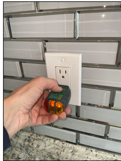
Not GFCI protected
