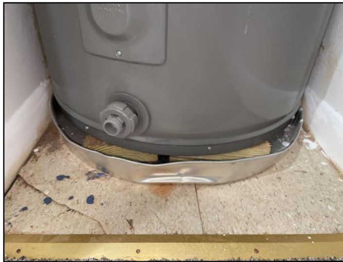
No visible drain on pan
