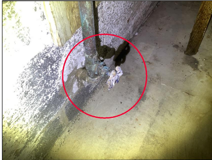
Corrosion water main valve.
