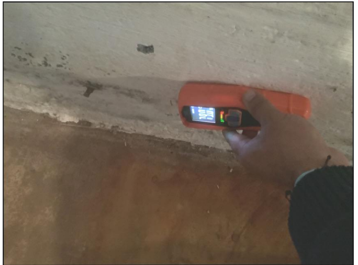
High moisture readings
