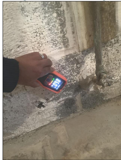
High moisture readings
