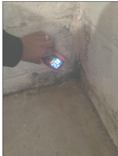
High moisture readings
